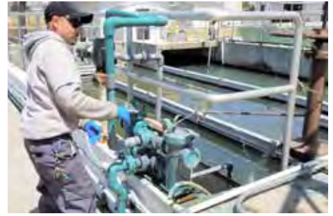
Operator Backflushing the Chlorine Analysis System.
