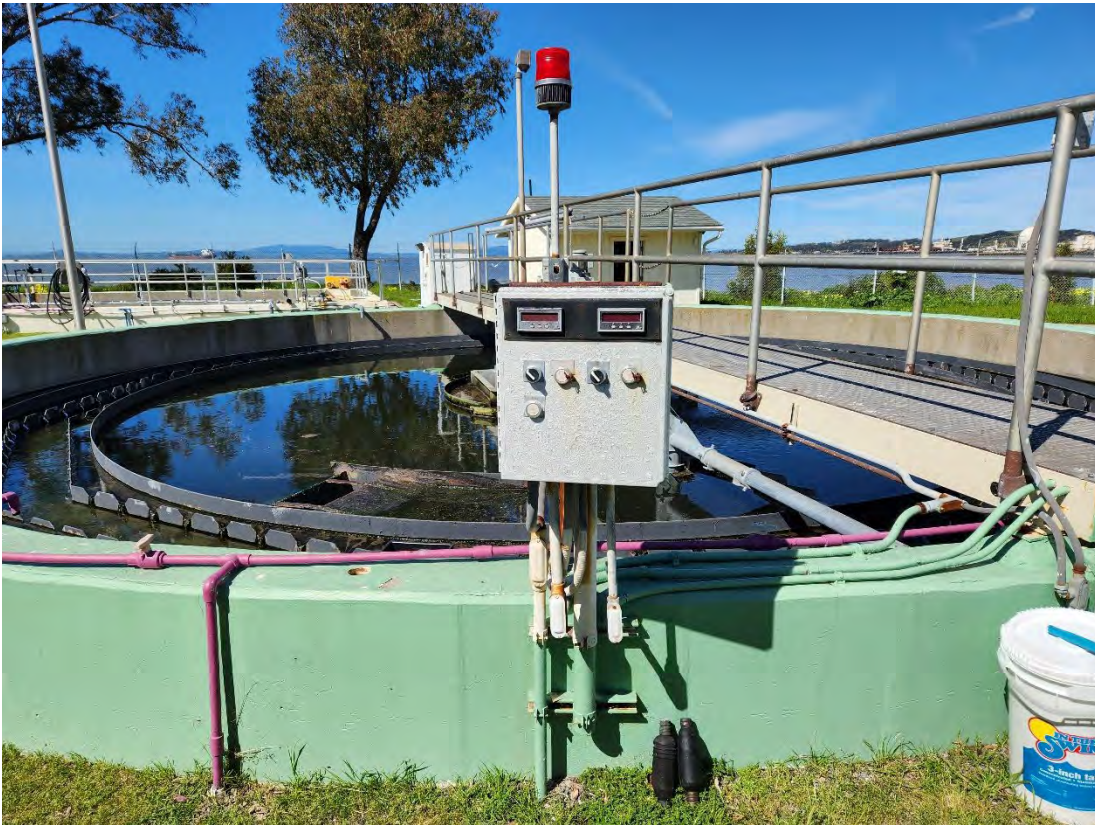
Single Local Control Panel for both clarifiers – not code compliant.
