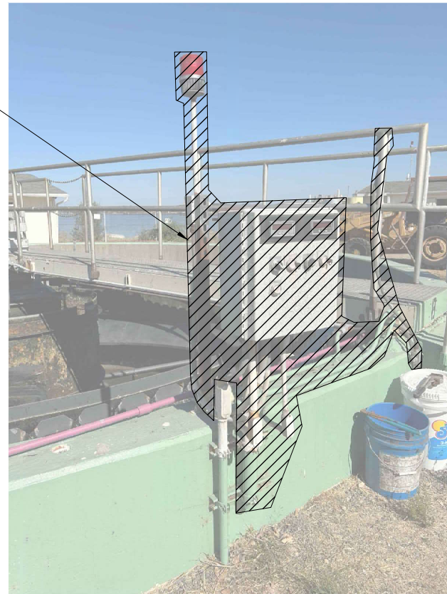
PHOTO - SECONDARY CLARIFIER ② SCALE: NO SCALE
