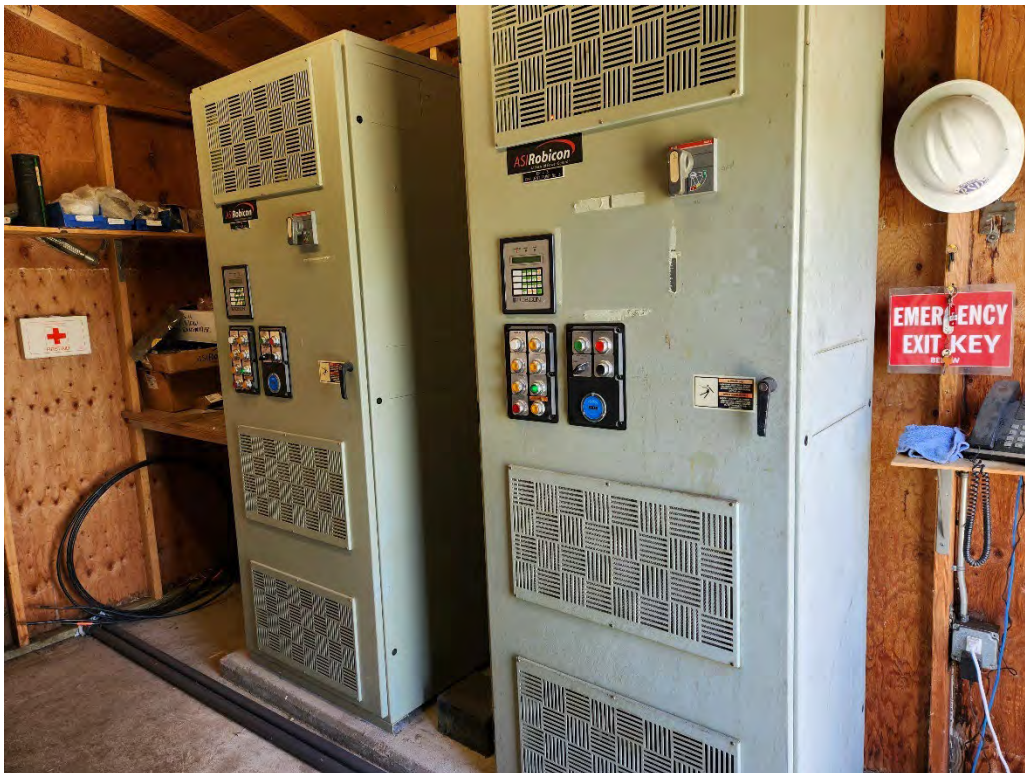
100 HP VFDs for large effluent pumps
