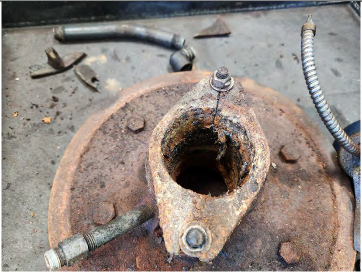
Severe Corrosion and crack
