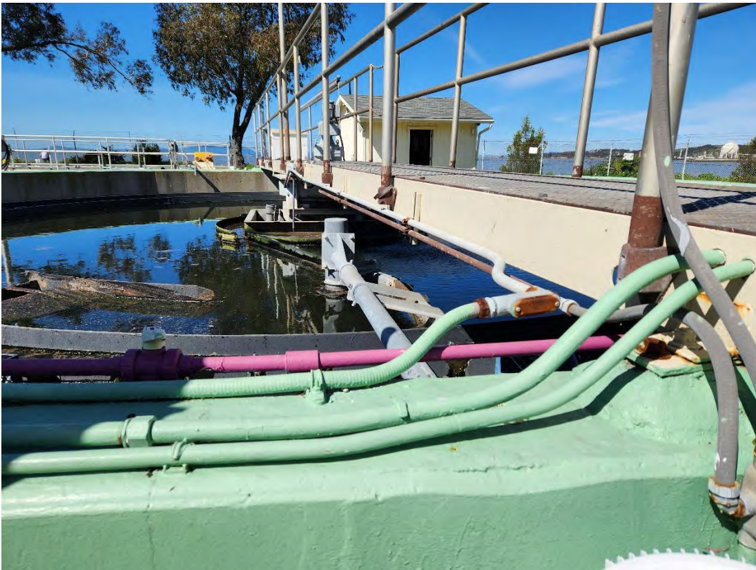
Maze of electrical conduits that may or may not be in use.
